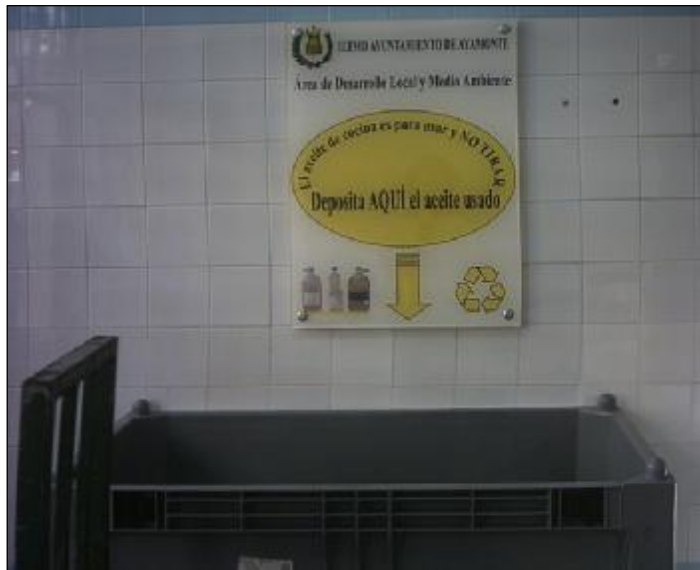
An example of Oil Bin installed in the City Market's back. Ayamonte.
